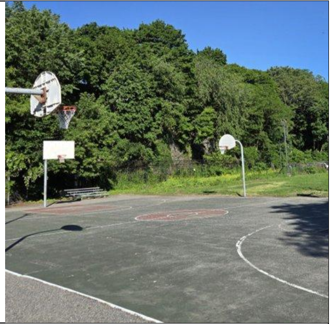
Photo 2: Existing basketball court surface showing deterioration
